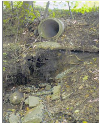
Figure 7: Erosion under outfall
